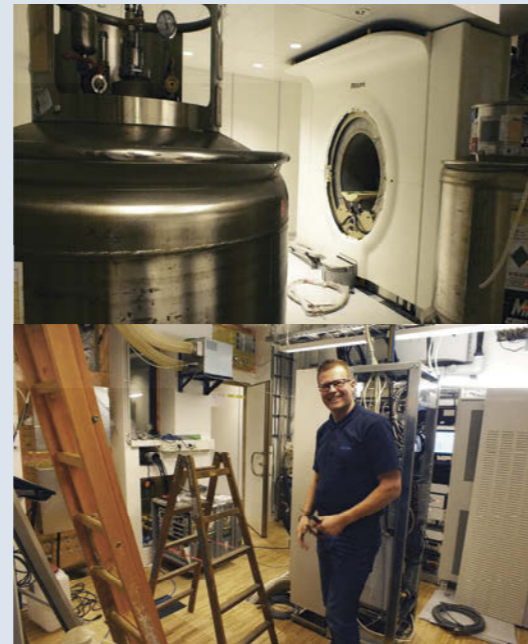
Photo 2: Philips engineer Klaus Rye installing the highly complex system. 5000 liter of liquid helium is used to keep the superconducting magnet at its working temperature of 4 Kelvin (-269 degrees Celsius).
