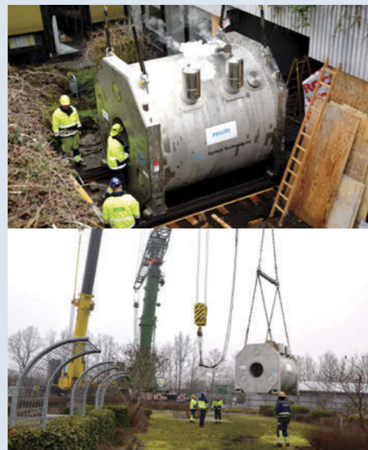
Photo 1: The big lift! The magnet was lifted and rolled to its current location on 1st of March 2014. Two of the strongest mobile cranes available in Denmark participated in this tandem lift of the 44000 kg heavy magnet.
